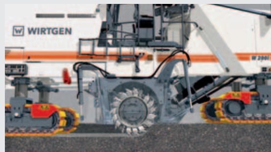
4 | The milling machine mills at full working depth right from the first metre
